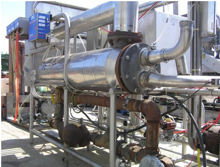
Figure 3 CIP System Shell and Tube Heater Reference Image
