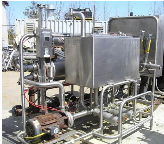
Figure 1 CIP System Motive Pump and Wash Tank Reference Image
